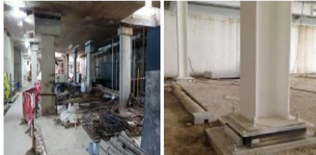
Fig. 3. Examples of the use of elastomer pads as vibration isolation for the structural elements [15]
