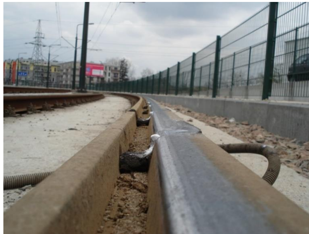
Fig. 6. Lube applicator through holes in the rail head on the tram curve in Krakow [14]
